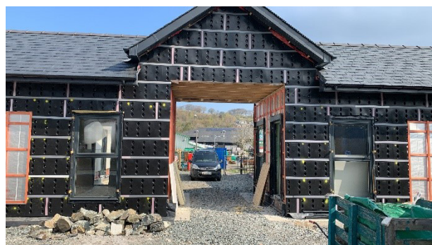
The former Ysgol Glan Wnion is about to receive a new stone face.
